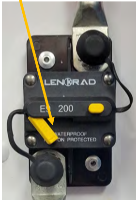
Circuit breaker OFF
